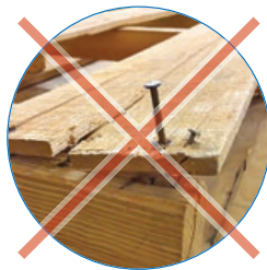
Raised nails greater than 1/8" are NOT ALLOWED .
